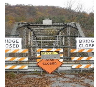
Inwood Bridge is closed to traffic, but will be restored.
